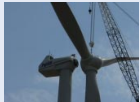
A propeller larger than the wingspan of a Boeing 747 is lifted by crane onto a wind turbine in Kimball, Nebraska.
